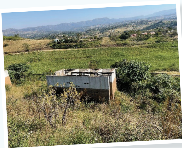
The learner toilets suffered extensive damage following the floods.
