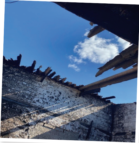
The remains of one of the administration blocks burnt during the riots.
